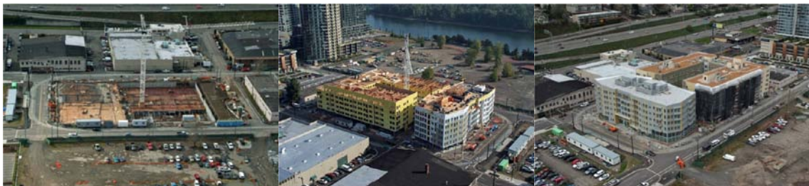
Figure 1: The MATISSE Apartment project in Portland, Oregon, United States completed in 2010 – Left: construction of 2-story underground reinforced concrete construction, Middle: 5-story wood frame over 1-story reinforced concrete with post-tension slab, Right: completed project. Photos: R&H Construction, General Contractor of the project.
